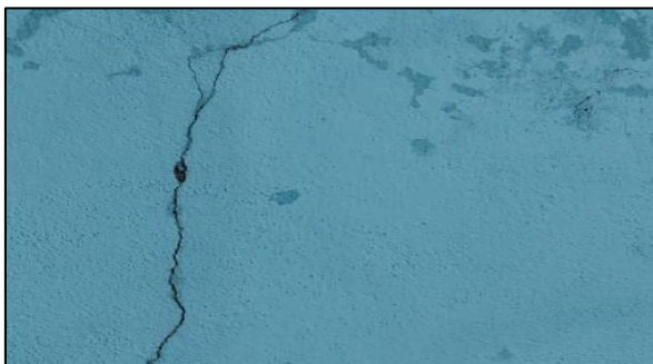
Fig.13 Crack on Structure
