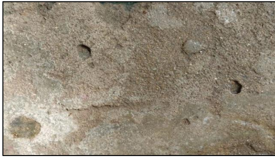
Fig.10 Pot Holes in Floor
