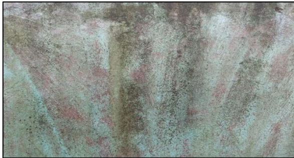
Fig.11 Small Holes in Wall
