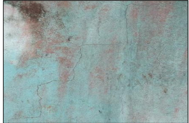
Fig.7 Cracks in structural elements
