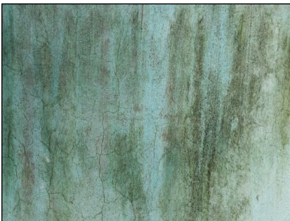
Fig.6 Stains and Hairline Cracks
