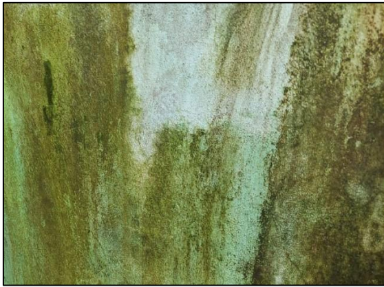
Fig.5 Stains in Structure
