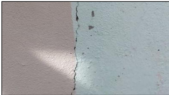
Fig.12 Crack on Joints
